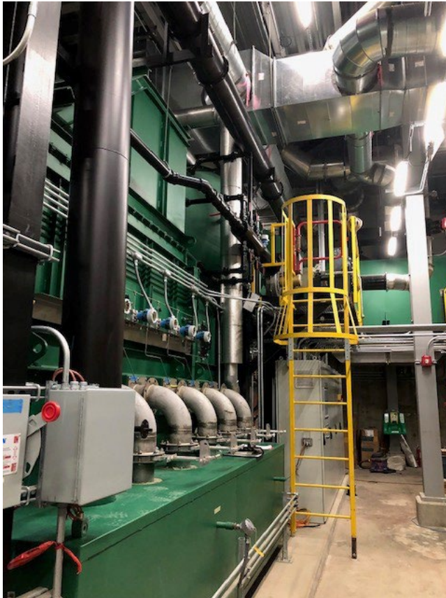
Gasifier Lower level
