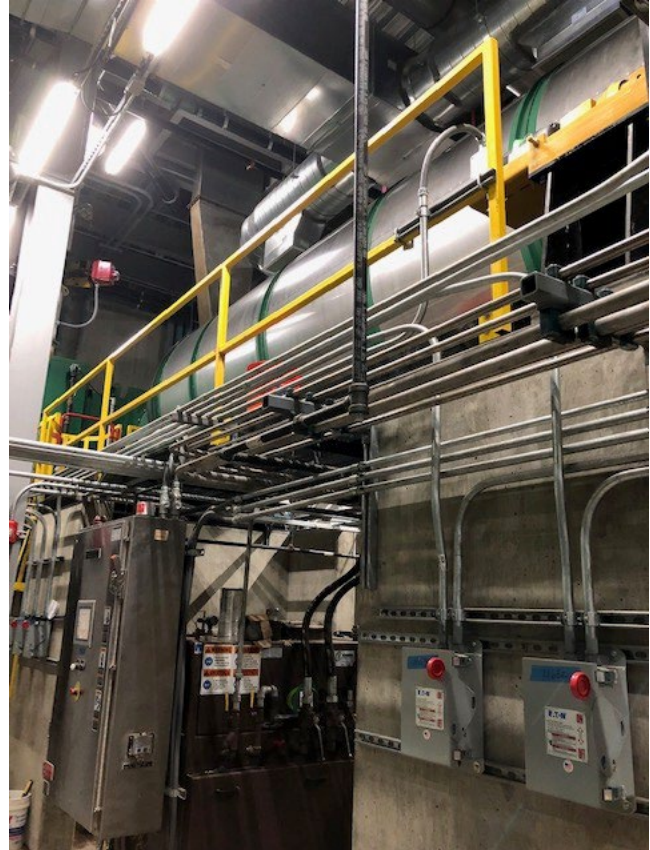
Dryer Lower level.
